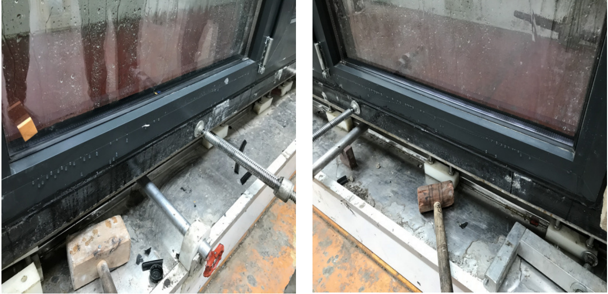
Photos 2&3. Water leakage (Test No: 2018.963.01 / 16.02.2018)
